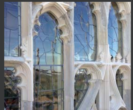
York Minster, Great East Window; largest example of medieval stained glass in England; external protection glazing with restauro®UV as stained glass with replicated lead lines; installation 2017
